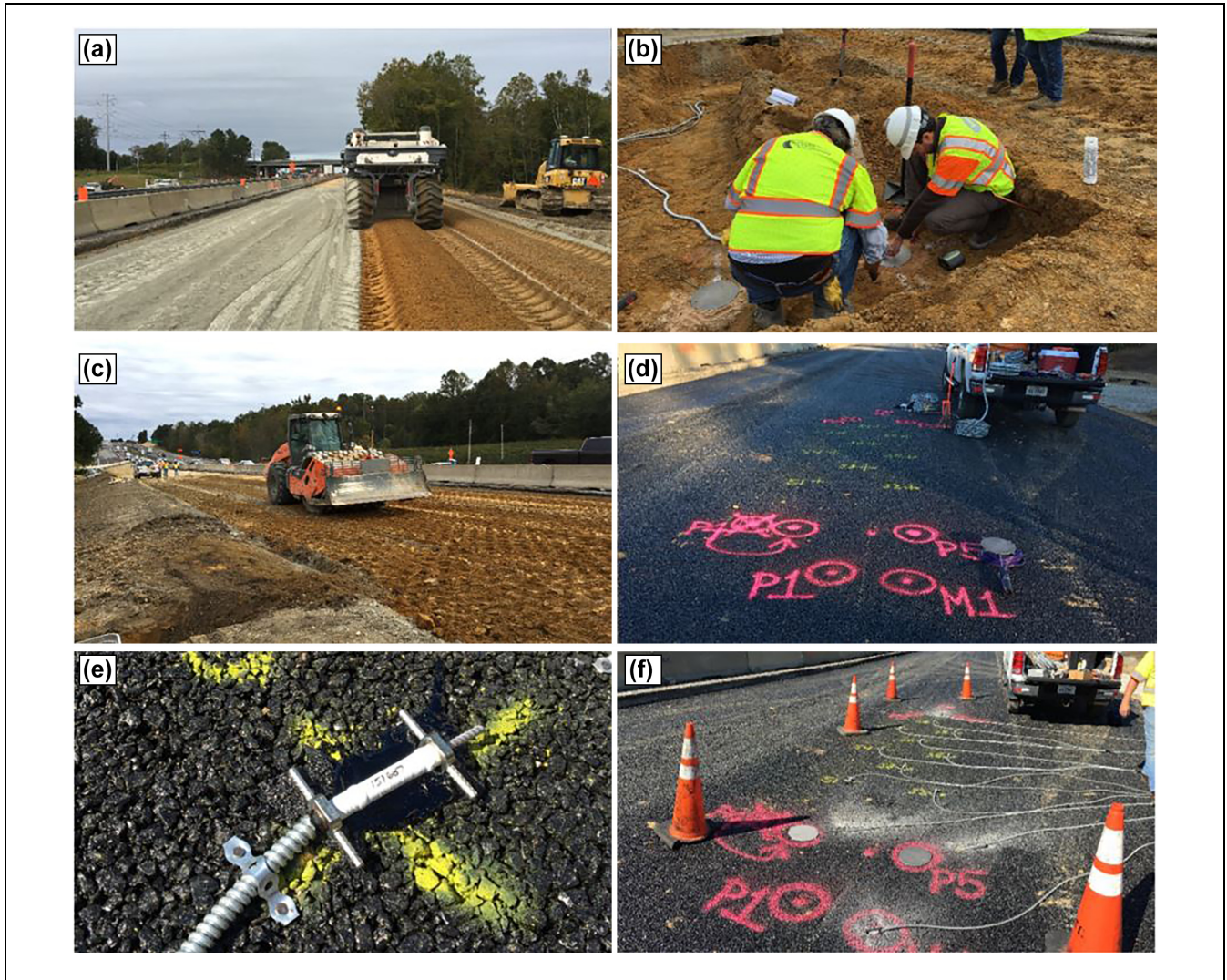
Figure 3. Instrumentation installation process: (a) full-depth reclamation placement, (b) installing sensors in trenched locations, (c) compacting full-depth reclamation over instruments, (d) marking locations on open-graded drainage layer, (e) close-up of strain gauge, and (f) completed array on open-graded drainage layer.
