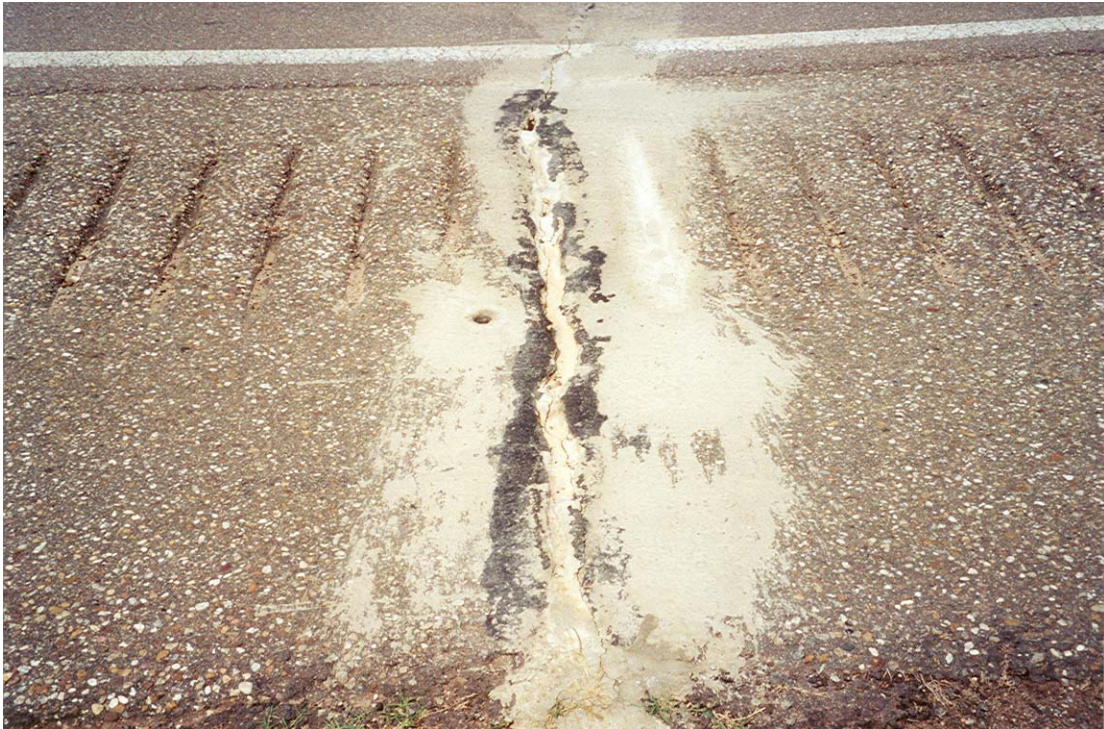
FIGURE 10 Treated transverse crack.
